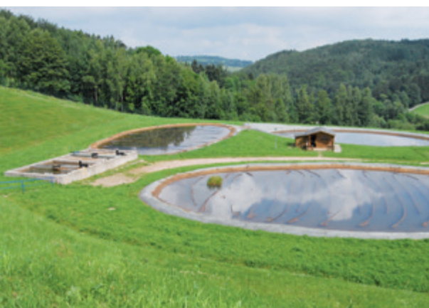
Fig. 10: Aerobically constructed wetlands
