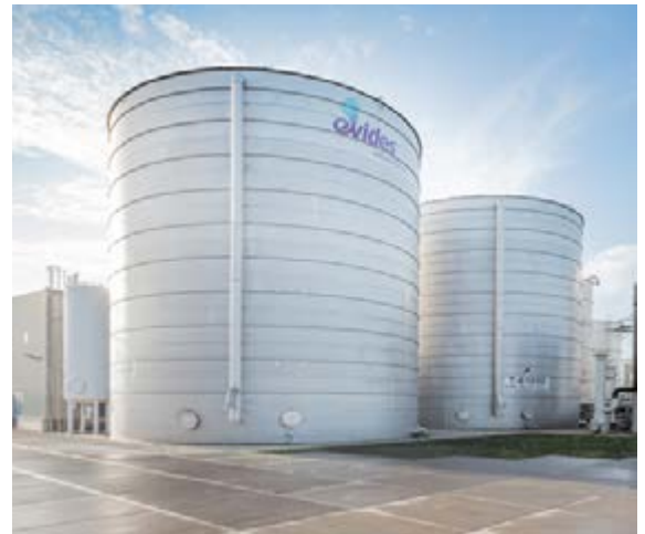
Demin water production Rotterdam NL, 2.100 m 3 /h
