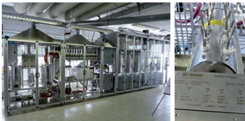
Fig. 32: Test facilities for developing catalysts for use in the reverse water-gas shift reaction for CO 2 activation; (2014 and 2015)
